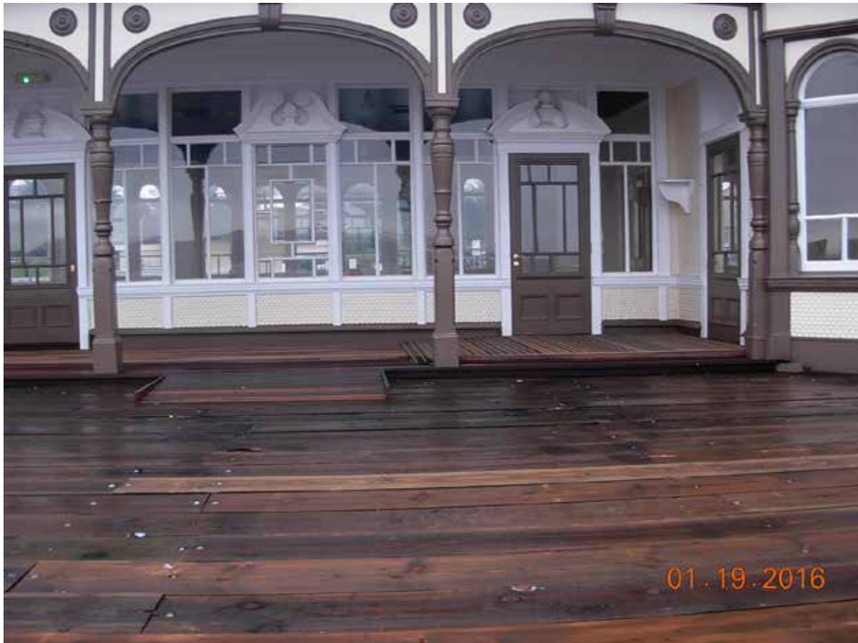
Waiting Room – January 2016. Veranda decking has been replaced and access ramps have been created to allow wheelchair access into the waiting room building. Decking is yellow balau and includes a resin/aggregate anti-slip application to the ramps and platform areas. Area of main decking in the foreground is awaiting application of Deckcoat anti-slip treatment.
