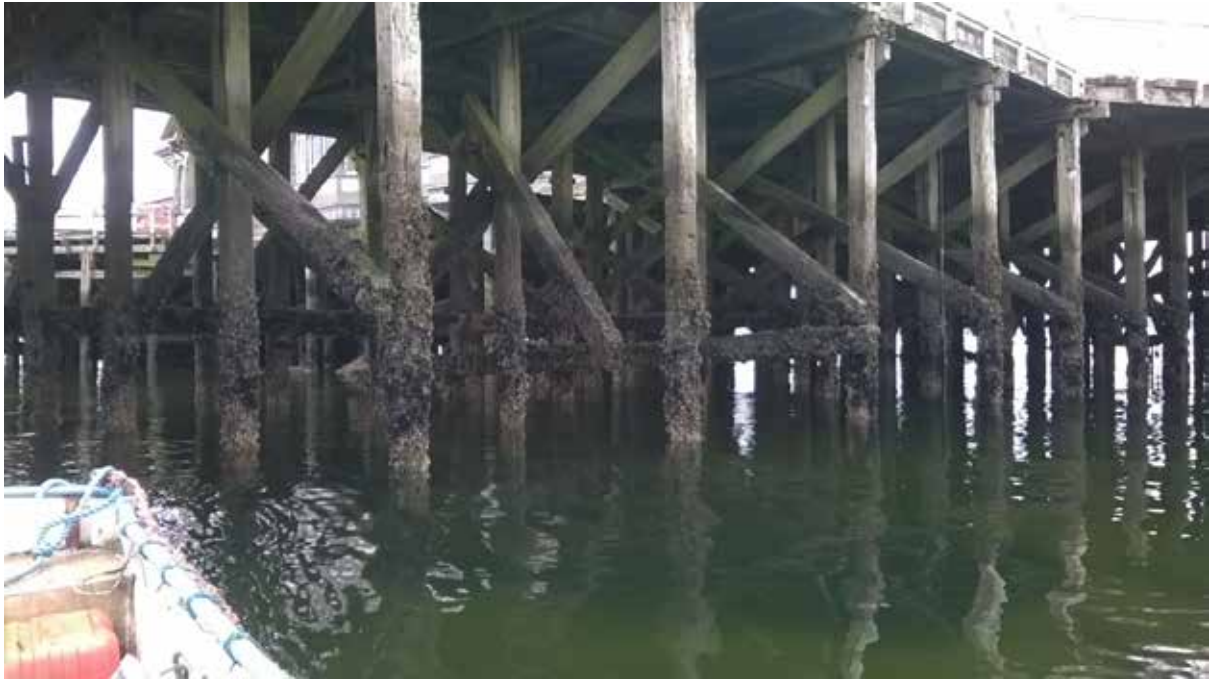
Structure of Pier – May 2014. Note longitudinal timber ties are missing to the foreground, diagonal timber braces are missing or no longer connected to the structure and timber columns are degraded
