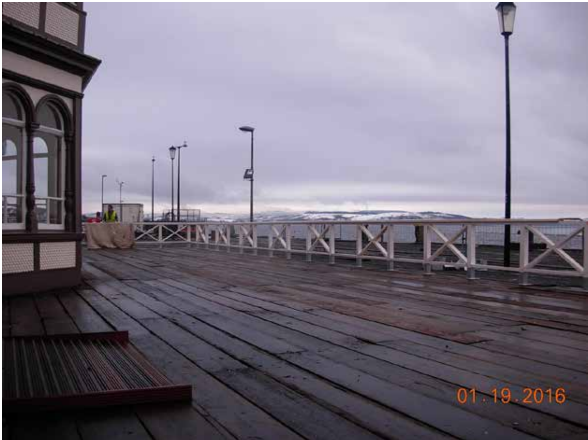
Pierhead – January 2016. Timber balustrade is being installed to demarcate the area that has been refurbished from the area which to be refurbished in Phase 2. The balustrade has been designed to the same specification and dimensions as the the original feature.
